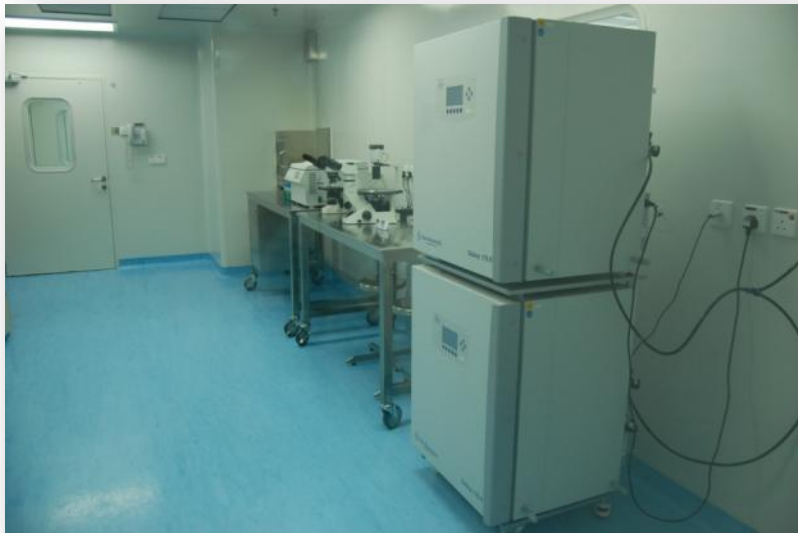
Equipments in CR1
